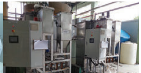
2 Sets of Pilot Plant of Moving Bed Biofilm Reactor (MBBR) Process
